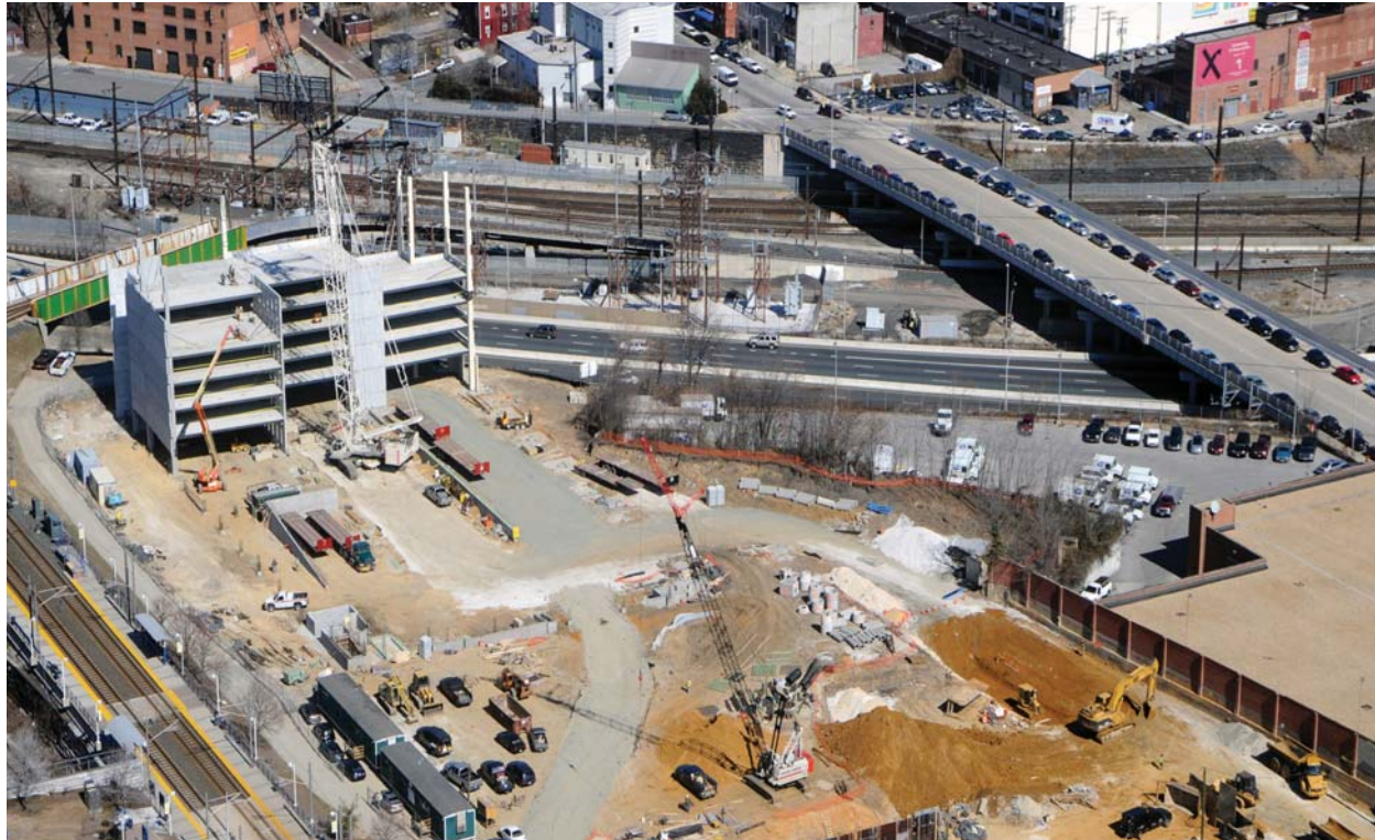
Viewed from above, the construction site of The Fitzgerald at UB Midtown is making considerable headway.
